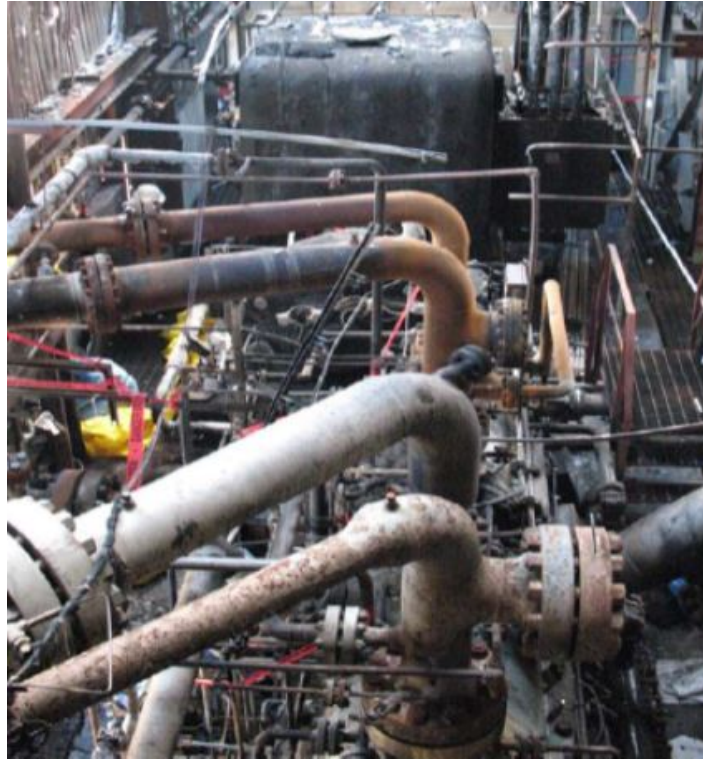
Fig. 1. Syngas compressor train
